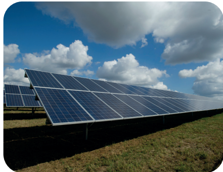
ENERGIE RINNOVABILI RENEWABLE ENERGY
