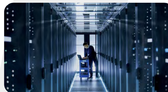
DATA CENTRE ECMWF Bologna - Italy
