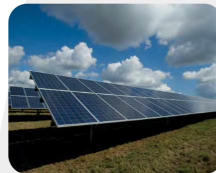
ENERGIE RINNOVABILI RENEWABLE ENERGY
