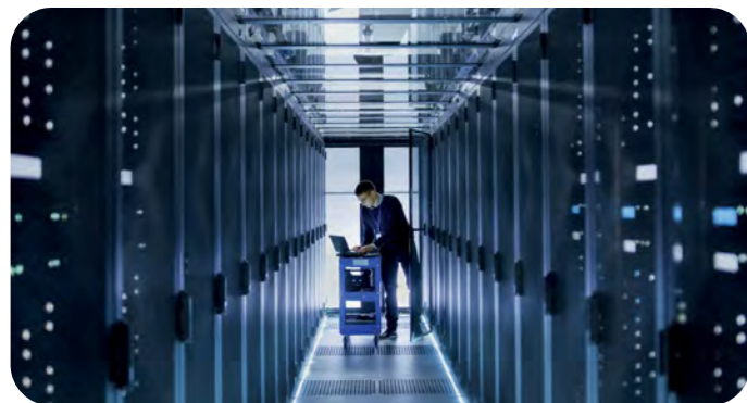
DATA CENTRE ECMWF Bologna - Italy
