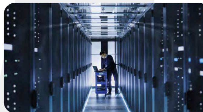
DATA CENTRE ECMWF Bologna - Italy
